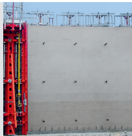
Only the tie holes and formlining joints are visible after using RUNDFLEX Plus-2.
