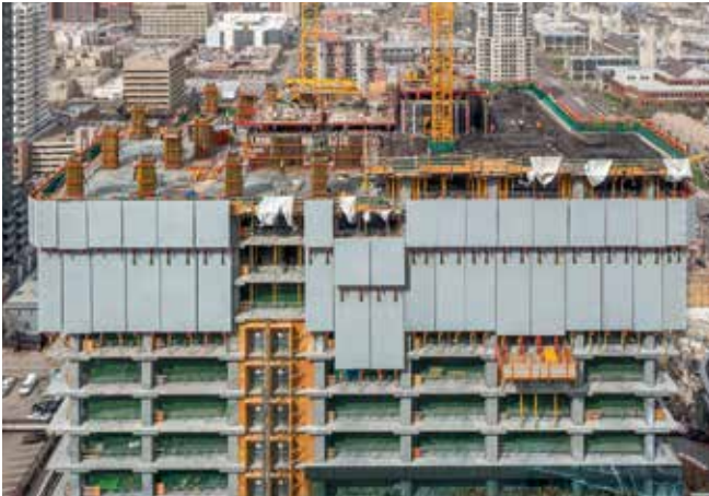
Tower ICE with 66 floors was built in the Ice District in Edmonton whereby the building core is being realized with the ACS Core 400
