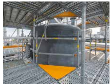
For gap-free scaffold installation of circular plant construction components with small diameters, the corner plate can also be used.
