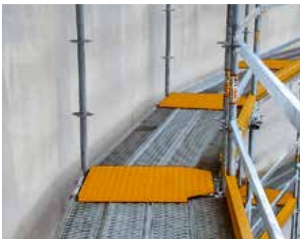
One cover plate is sufficient to cover the gaps in the decking of the rotated scaffold bays irrespective of the diameter of the circular structures.
